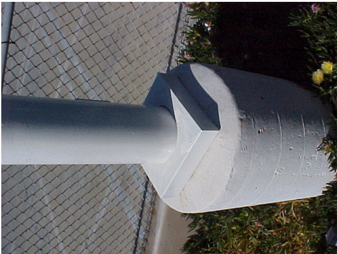
Base of existing light pole showing comparison of size between pole (9" dia.) and base (24" dia.) which demonstrates the approximate difference between the existing and the modified light pole
