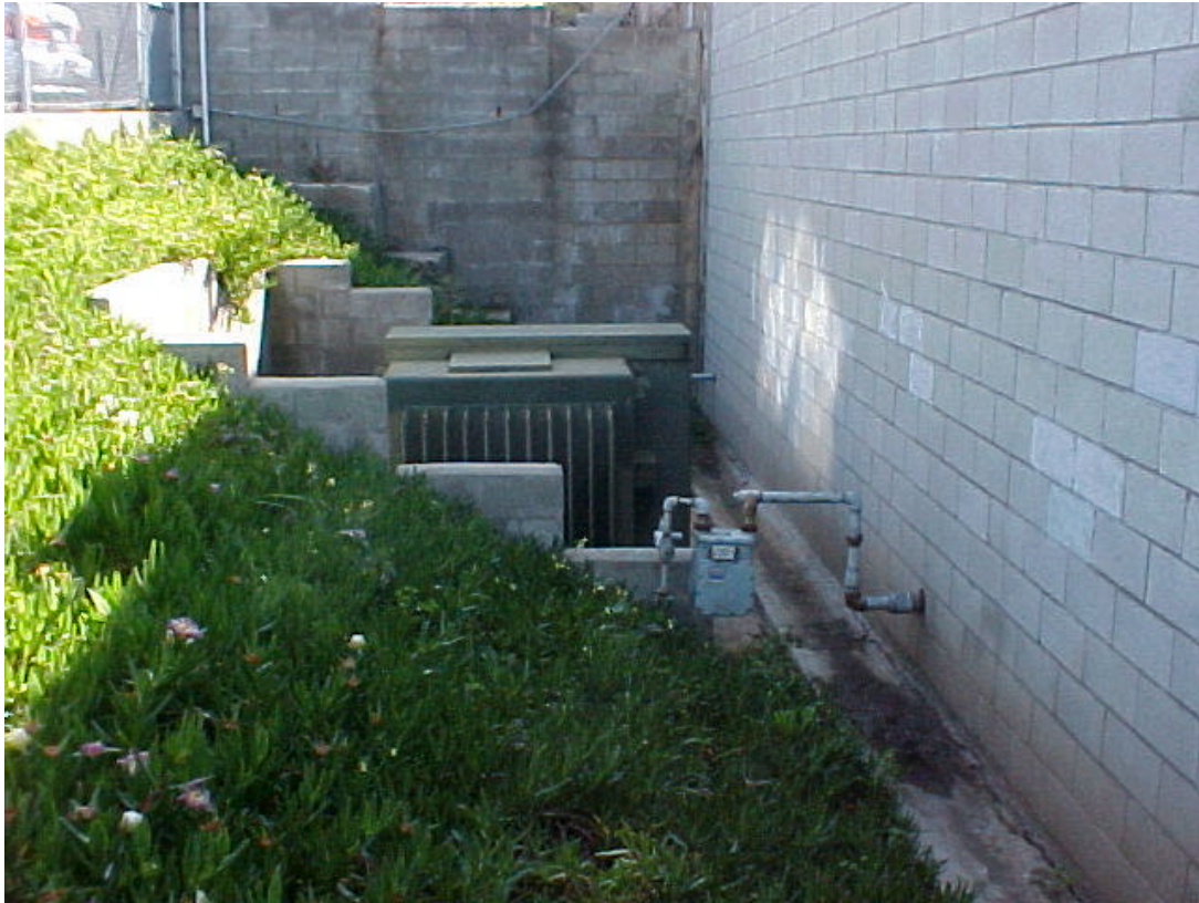
Location of existing transformer and proposed wireless telecommunications equipment cabinets
