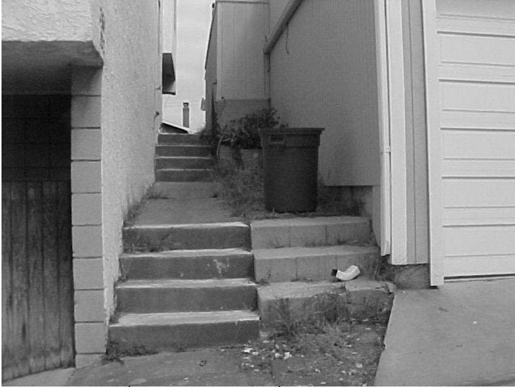
Rear grade from 33 rd Place between 242 33 rd Street and property to the west
