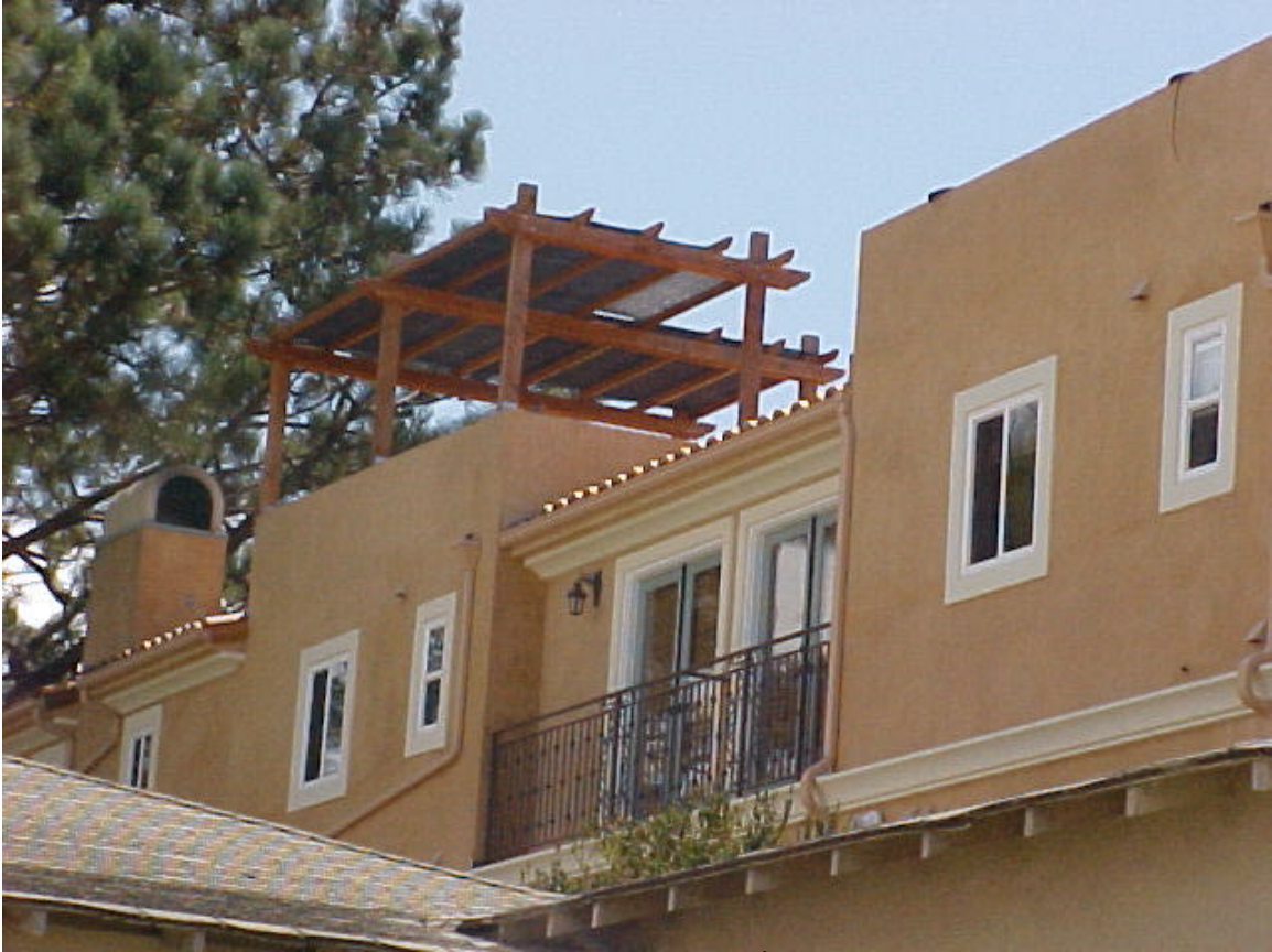
August 13, 2003 – Over-height shade ramada at 506 11 th St. owned by the Nelsons.
