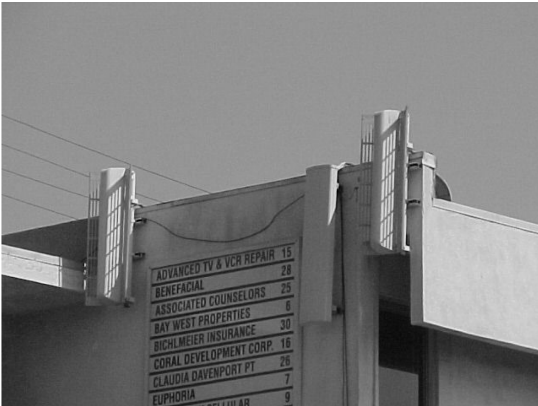
Close-up view of existing antennas mounted on the building's north façade
